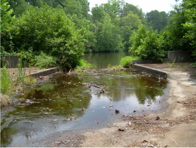
Figure 1. Concrete spillway. It looks in good shape and almost free of debris.
